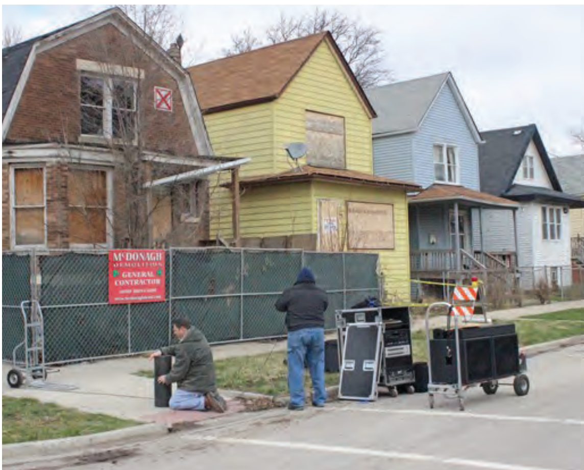
Figure 19: A vacant home being prepared for demolition in Chicago's Englewood neighborhood. Source: dnainfo.com
